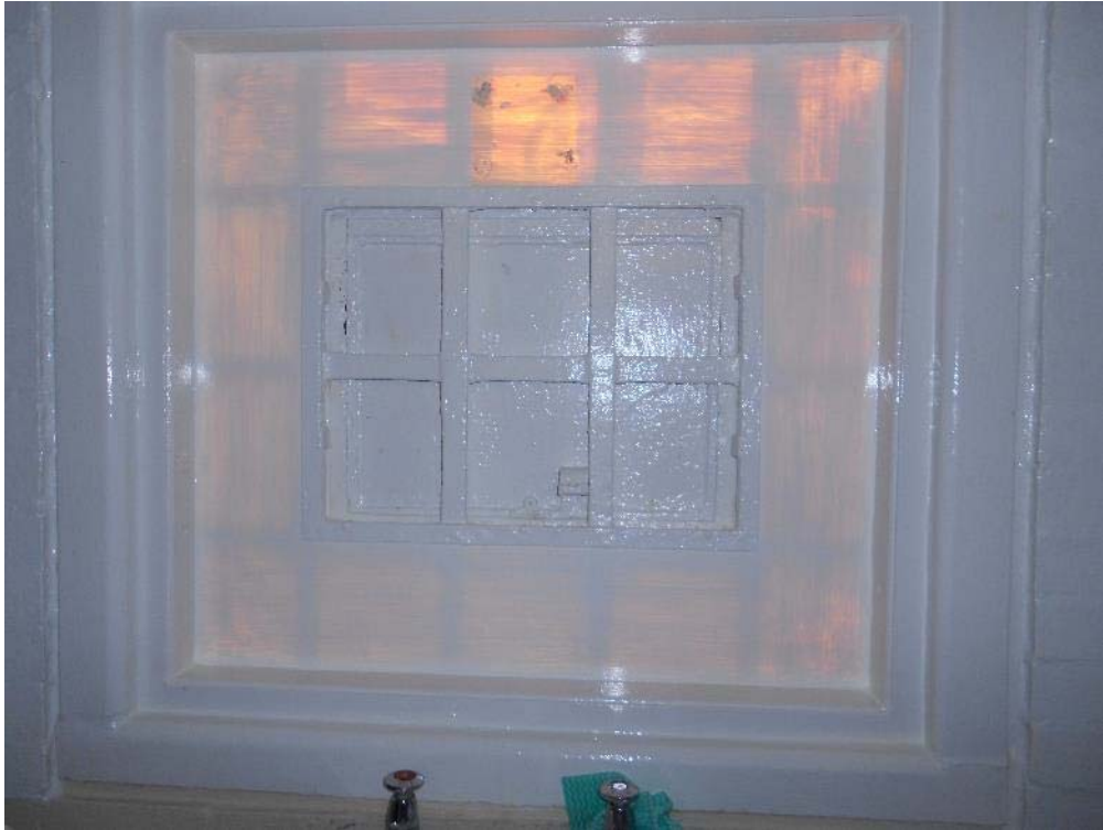
Painted over cell window on A wing
